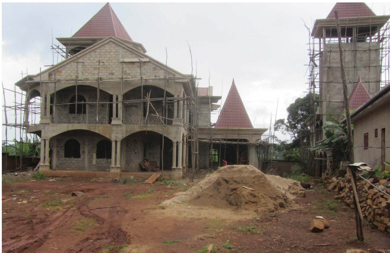
Family house under construction in a rural village, Bamboutos, Cameroon. Housing materials are an important household expenditure from remittances © Paul van Lindert
